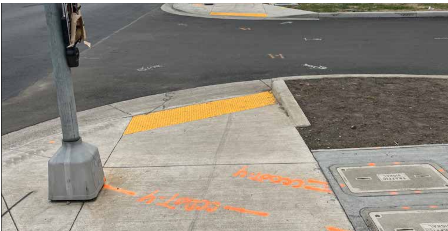
The work still underway includes finishing the pedestrain signals and lane markings.
